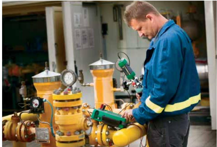
Periodic calibration of instruments is required. The typical process parameters calibrated at plant Łódź are related to delivering natural gas.
