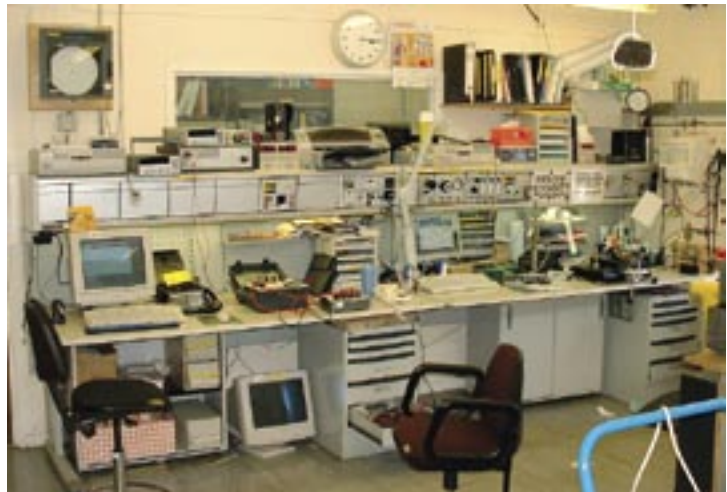
The workshop utilizes a Beamex calibration bench system with panel-mounted calibrators.
